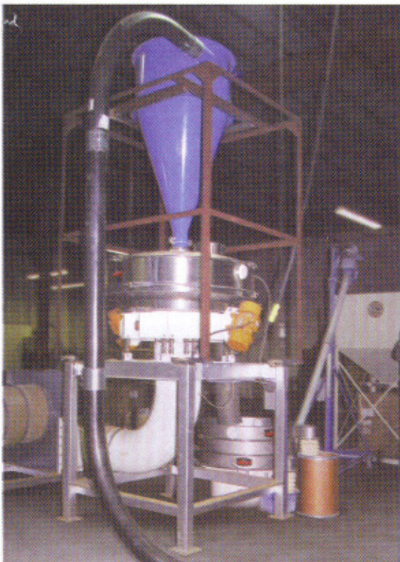
Cellulose plastic pellets move from a pelletizer to a cyclone separator via a pneumatic conveyor. They are gravity discharged into a 60" dia. circular vibratory cooler that reduces their temperature to 100°F (38°C) and moisture content to less than 1 percent.
